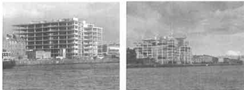
Figures 5 & 6: The large unfinished Anglo Irish Bank building on Dublin's Quays: A visual reminder of the boom and bust era. Among proposals for the redevelopment of this site was a vertical garden.
